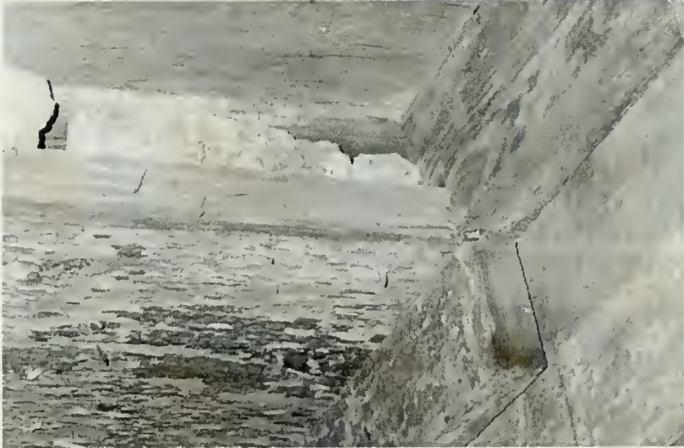
Figure 25 Close-up of “Palling” under the floorboards in the Basement of the South Wing of the Main House, 2002
